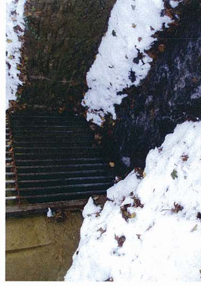
Fall: View looking down the steep bank at Station 3, the grated discharge under Carlton Avenue.
