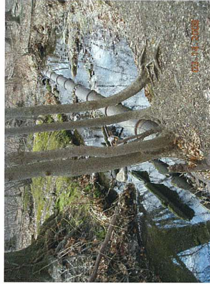
Spring 2008: Sewage pipe remnants next to active sewage line running through Stannards Brook.
